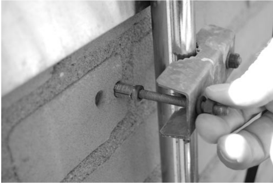
(a) The wind loosened a peg of an antenna mast mount.
